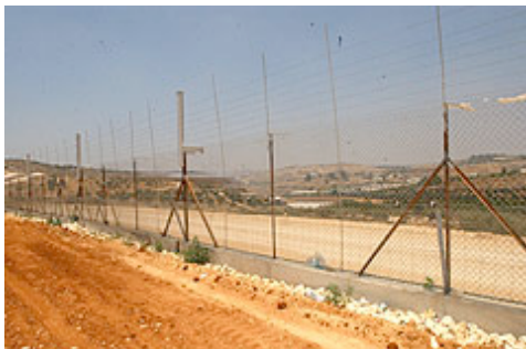
Intrusion detection fence
